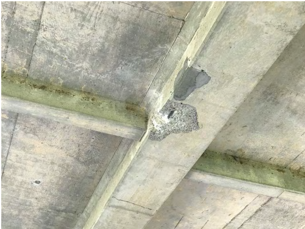
Closeup of damage under bridge
